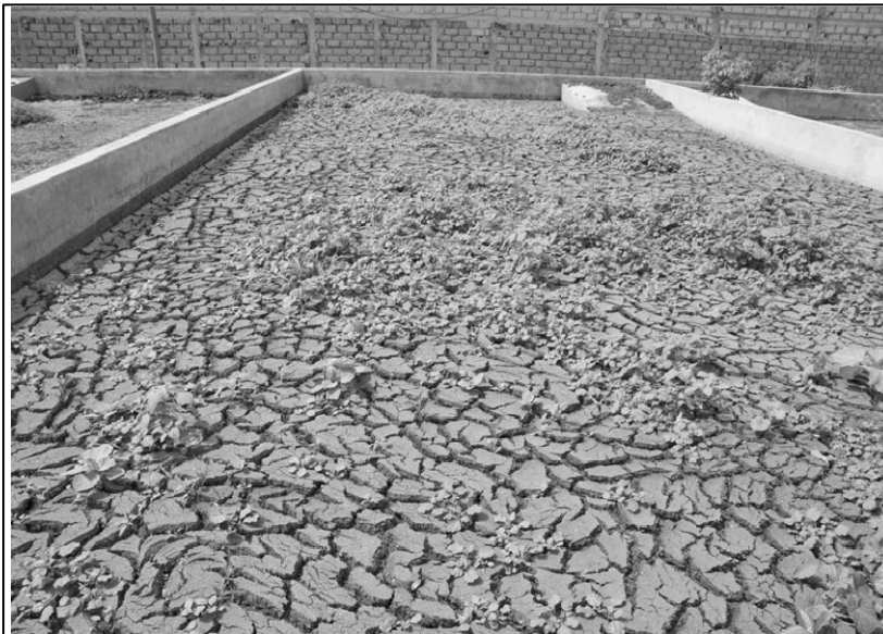
Figure 4 Faecal sludge drying bed currently in operation at Cambéréne Faecal Sludge Treatment Plant in Dakar.
